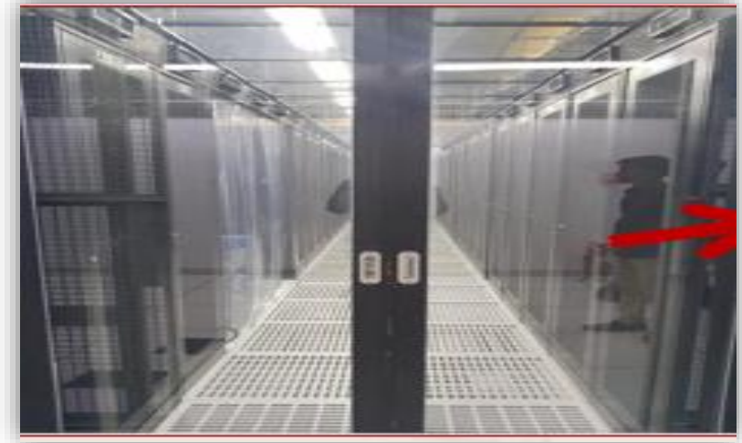
Server Room Cold Aisle containment
