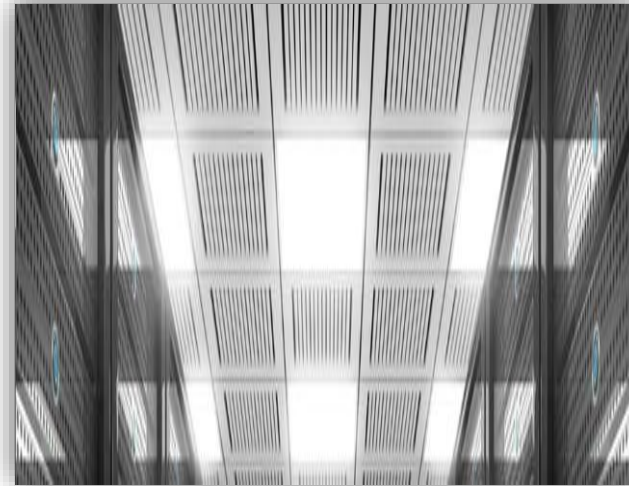
Server Room Led Light
